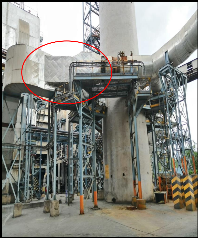
Hot gas duct from TPP
